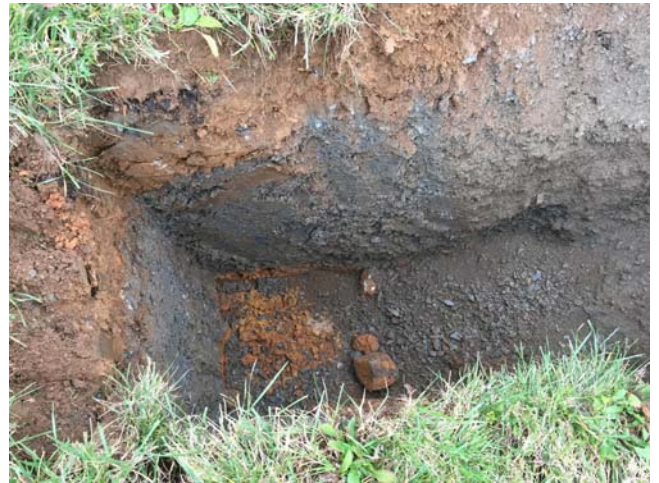
Photo 10 – TP-5 – Trace amounts of asphalt (upper left side of the excavation) and apparent CR6 underlain by natural soils
