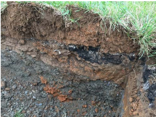
Photo 11 – TP-6 – Asphalt material and apparent CR6 underlain by natural soils
