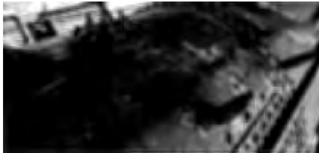
The mounting flange for the check valve, and brackets of the feedwater pipes.
