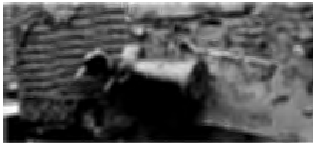
Loose handrail stanchion.
